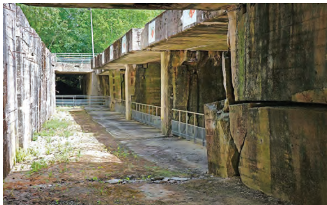
Trackbed of what was to be the fortified train station, transit halls to right. Photo Bob Clary
